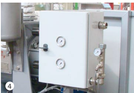
Pneumatic control panel
